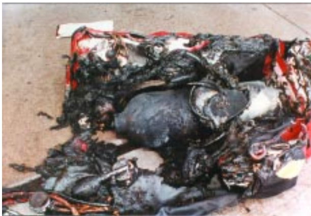
Damaged Oxygen System
