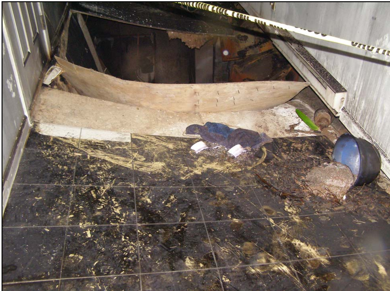
Photo 2: Depicts the failed floor from above. Note the front door in the upper left-hand corner. Photo courtesy of the fire department.
