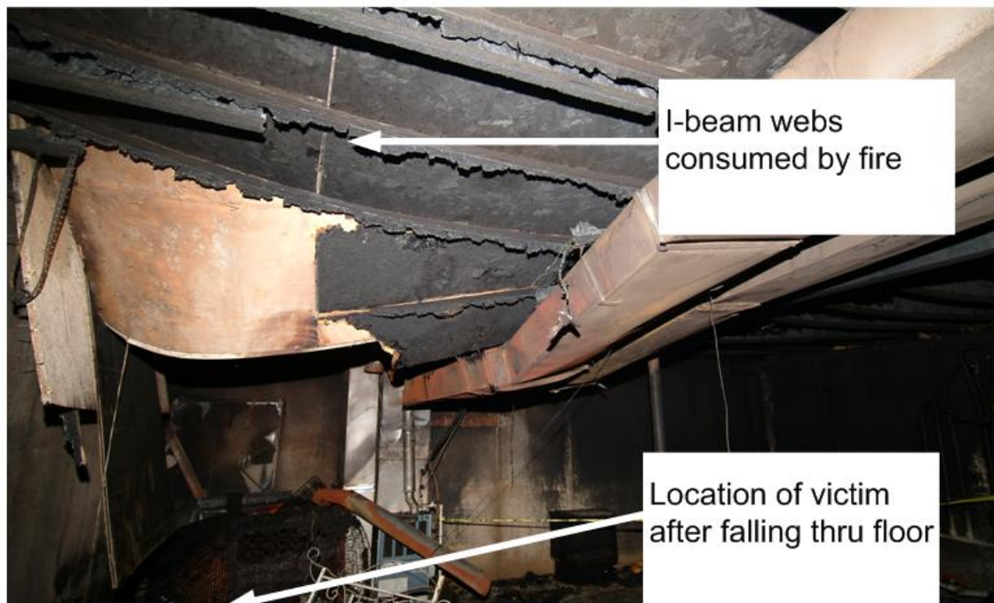
Photo 3 illustrates the floor failure area, viewed from the basement. Photo courtesy of the fire department
