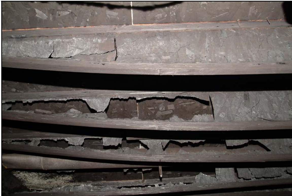
Photo 5: Depicts the significant damage suffered by the webbing of the I-joists as compared to the flanges. This damage resulted in floor instability and failure. Photo courtesy of the fire department.
