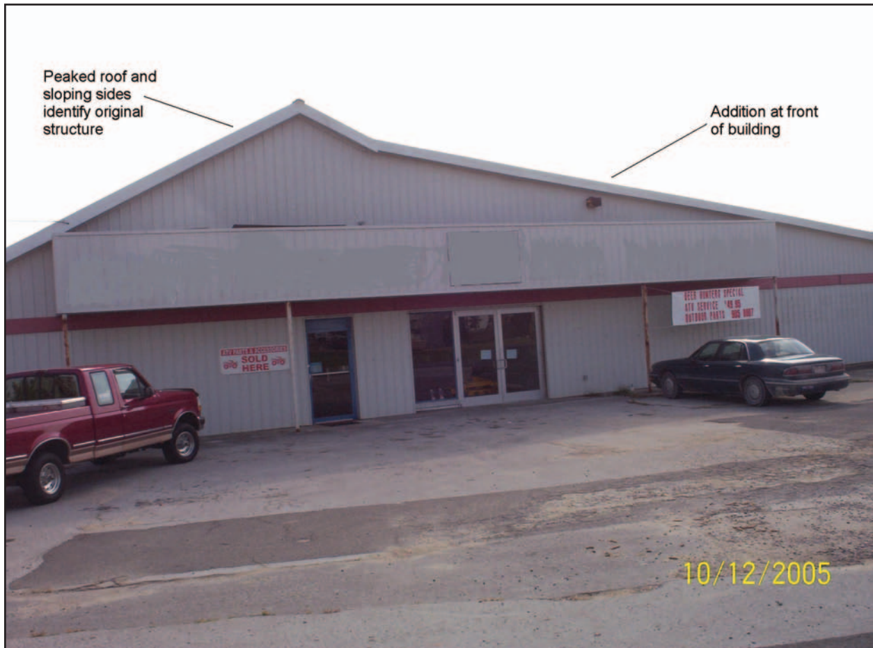
Photo 1. Photo taken four months prior to the incident. Note the front of the building and the awning over the entranceway. The sheet metal siding completely hides the presence of the underlying concrete block wall covered over with brick veneer and wooden clapboard siding. At the time of the incident, a large lighted sign was mounted on the awning above the entranceway. Photo courtesy of state fire marshal's office.
