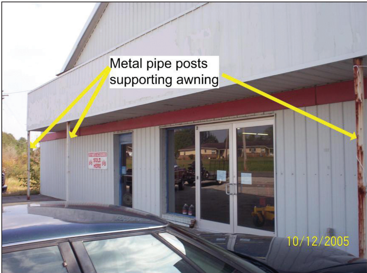
Photo 3. Photo of A-side of the structure taken four months prior to the incident. Note the overhanging awning over the entranceway. Note the metal pipe posts supporting the front of the awning. A total of 4 metal pipe posts supported the awning. Photo courtesy of state fire marshal's office.
