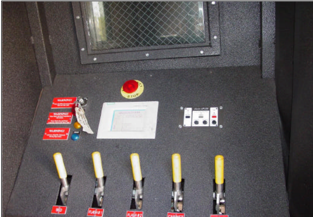
Photo 2. Operator control panel. Individual gas control valves are shown at the bottom
