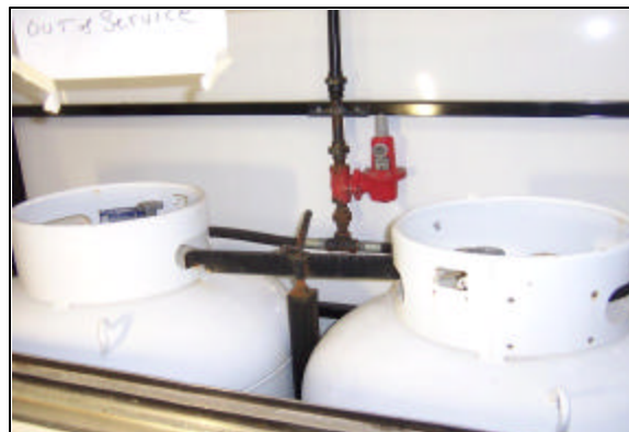
Photo 3. LPG cylinders in equipment room at front of trailer.
