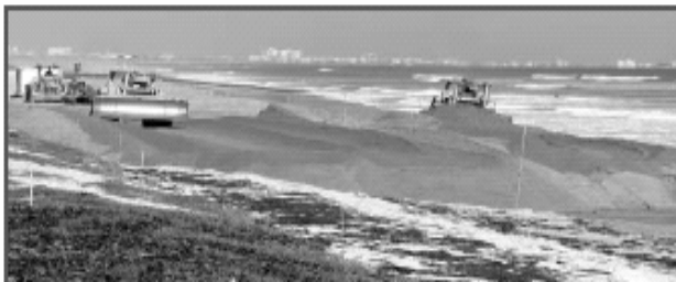
Figure 13: Restoration efforts using OCS sand resources on Patrick Air Force Base near Coca Beach, Florida.
