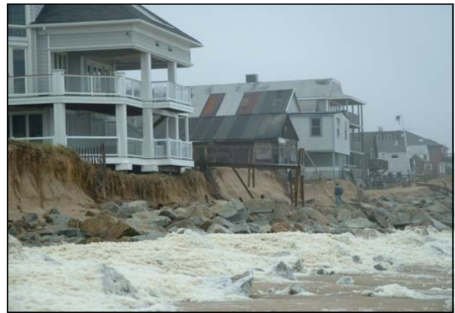
Coastal erosion along Massachusetts’ North Shore after the Patriot’s Day Storm. Photo courtesy of MACZM
