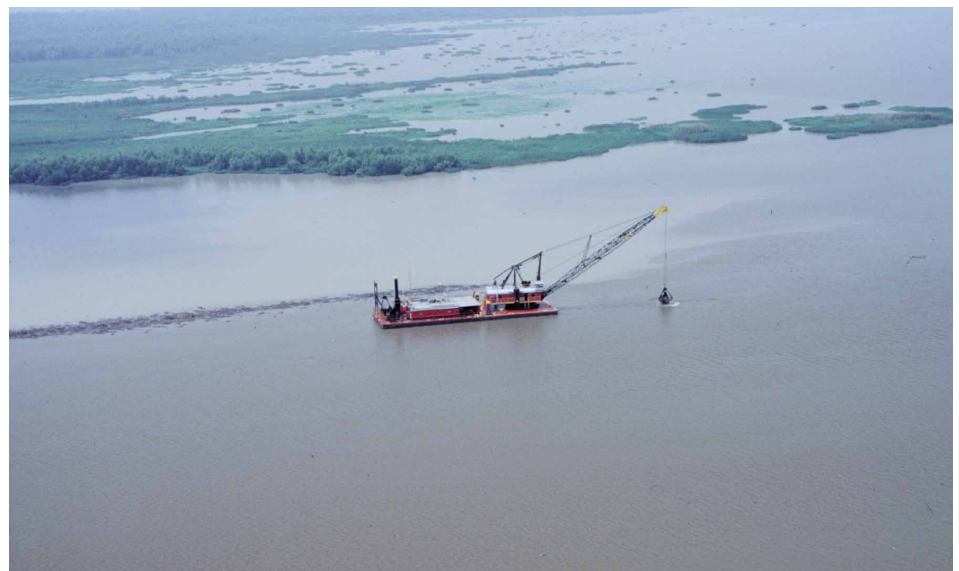
▲ Figure 3. Bucket dredge, Capt. Bufford Berry, constructing containment levee in Atchafalaya Sediment Delivery site. (Photo courtesy of Dr. Erik Zobrist, NOAA Habitat Restoration.)
