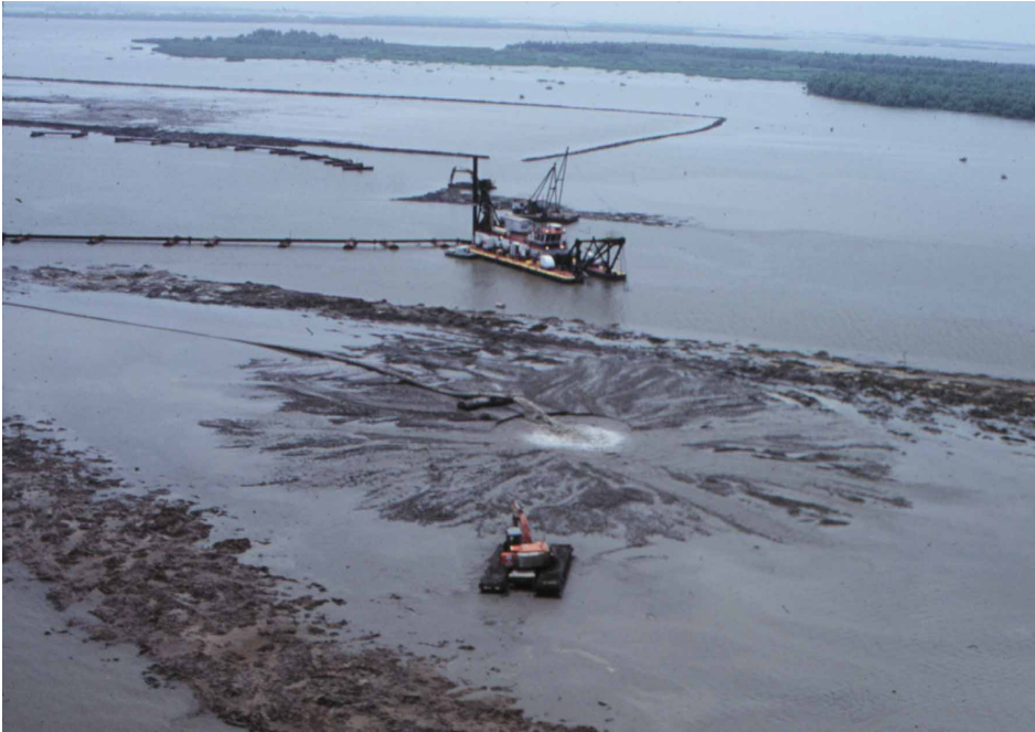
▲ Figure 2. Hydraulic dredge Katrina pumping material into containment area on Big Island project site. (Photo courtesy of Dr. Erik Zobrist, NOAA Habitat Restoration.)
