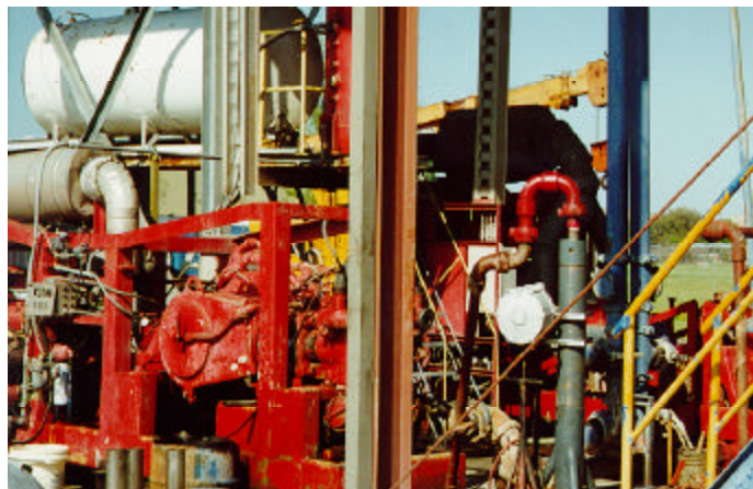
Figure 34: Photograph of Pump and Test Stand
