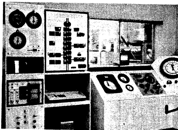
Fig. 8—Instrumentation panels in control room.
