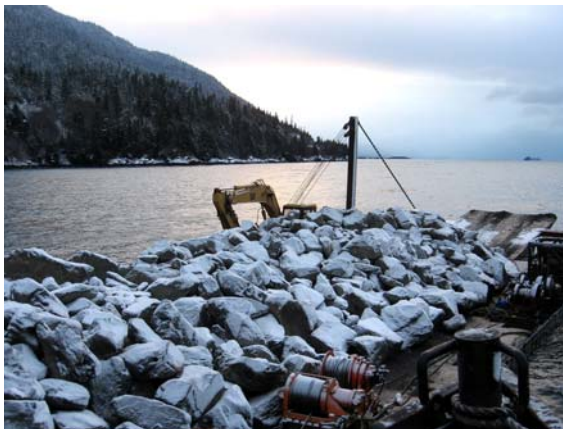
Figure 2: The barge loaded with rock ready to travel to the construction site. Rock sources were Juneau's Hidden Valley and excess rock from roadbuilding at the Lake Dorothy hydropower project in Taku inlet.
