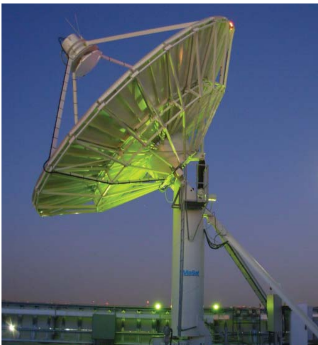
A satellite antenna at the NOAA Satellite Operations Facility (NSOF)
