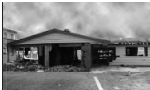
Storm surge can cause substantial damage to unprotected buildings.
