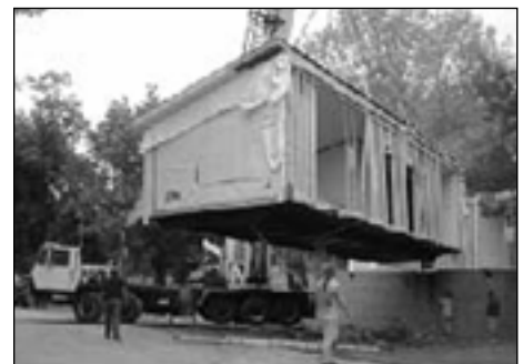
Glaze home being lifted into place 8' above the ground. (Photo by Anita Nance)
