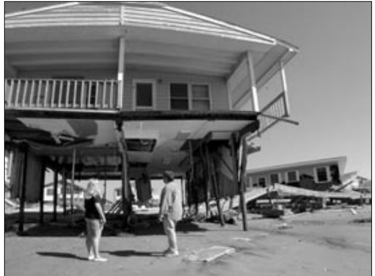
Mark and Angela Godfrey survey the damage to their North Carolina beach home after Hurricane Floyd struck. (Photo by Dave Gatley, FEMA)
