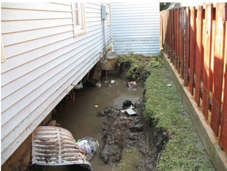
Figure 1: An example of a caved in basement wall due to the force of the rushing water.
