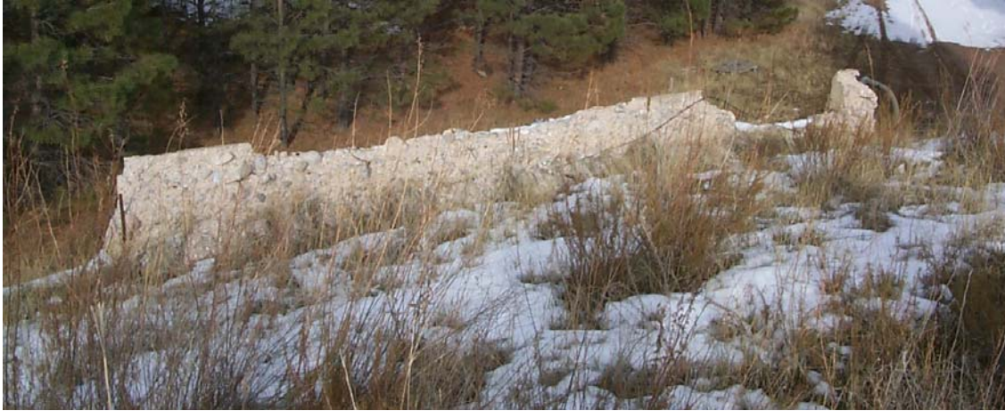
Figure 13b. TA-8-1, concrete spalling at parapet, looking northeast
