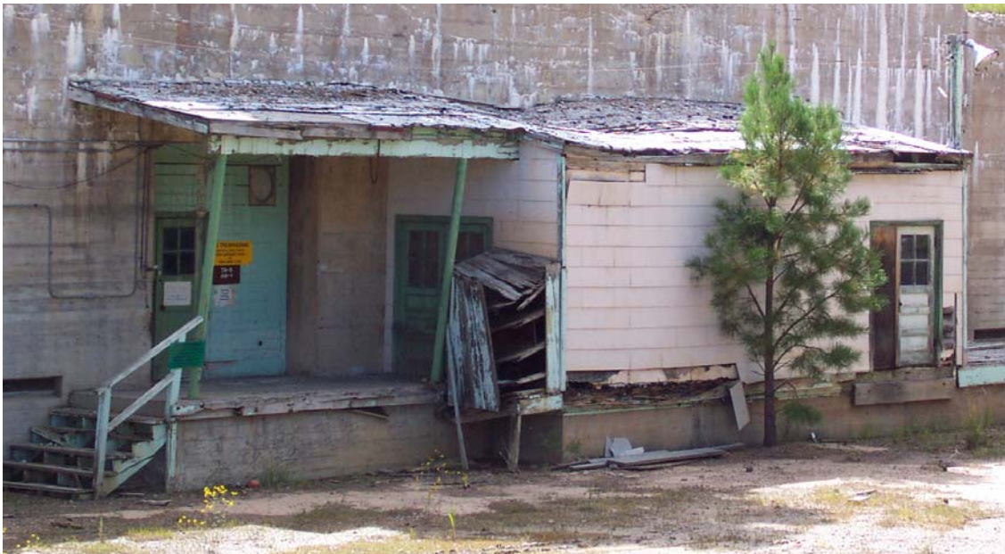
Figure 9. TA-8-1 (entrance steps and wooden canopy to be replaced at left; deteriorated dock addition, storage bins, and tree to be removed at right)
