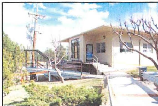
Photo 1e: Detail view of north entry vestibule and metal stairs to lower entrance
