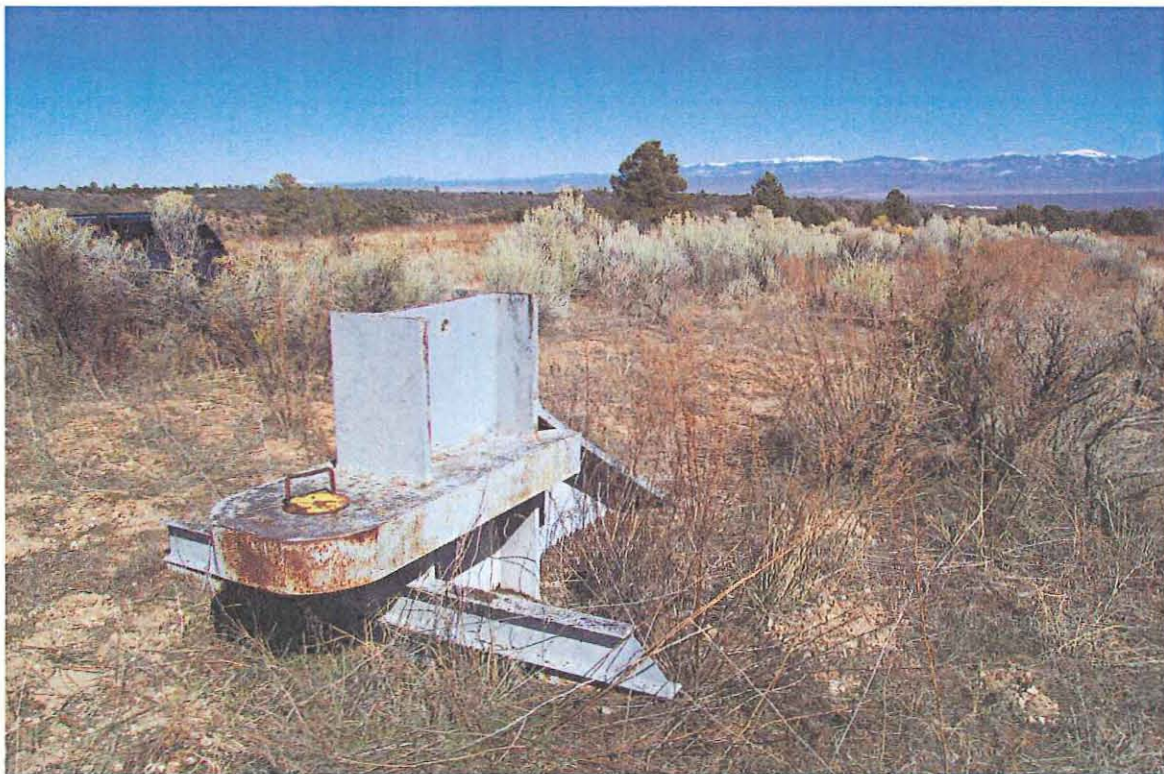
Anchor (above ground portion) located to the east of TA-49-121 Cable Test Facility, direction northeast (2005)
