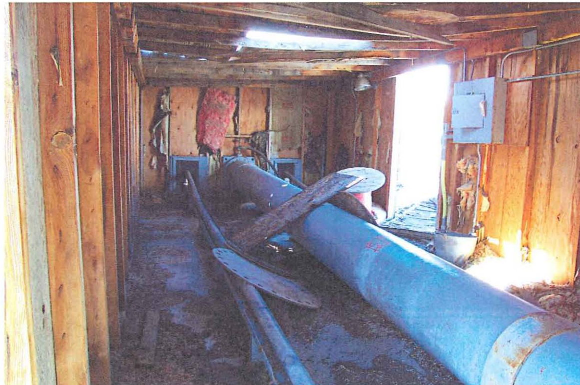
TA-49-121, Hydraulic Ram Enclosure, direction northwest (2005)
