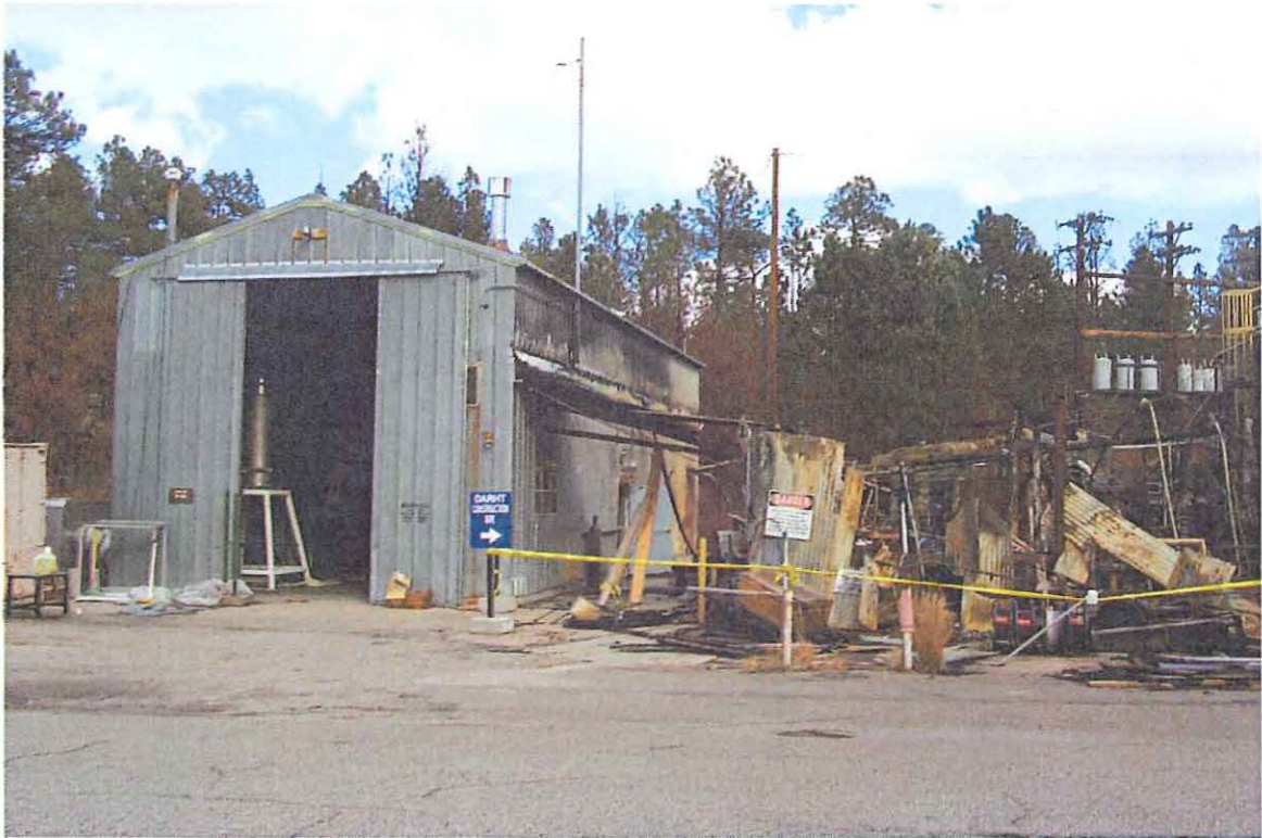
TA-15-194, south and east sides, direction northwest. East side connected to a covered passageway that burned in the Cerro Grande Fire May 2000.
