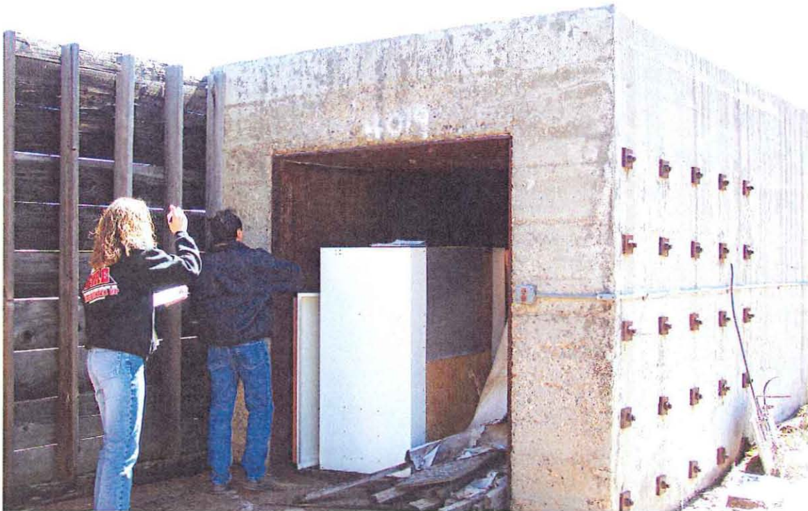
TA-6-9, Northeast wall and northwest wall of southern portion of building, direction south
