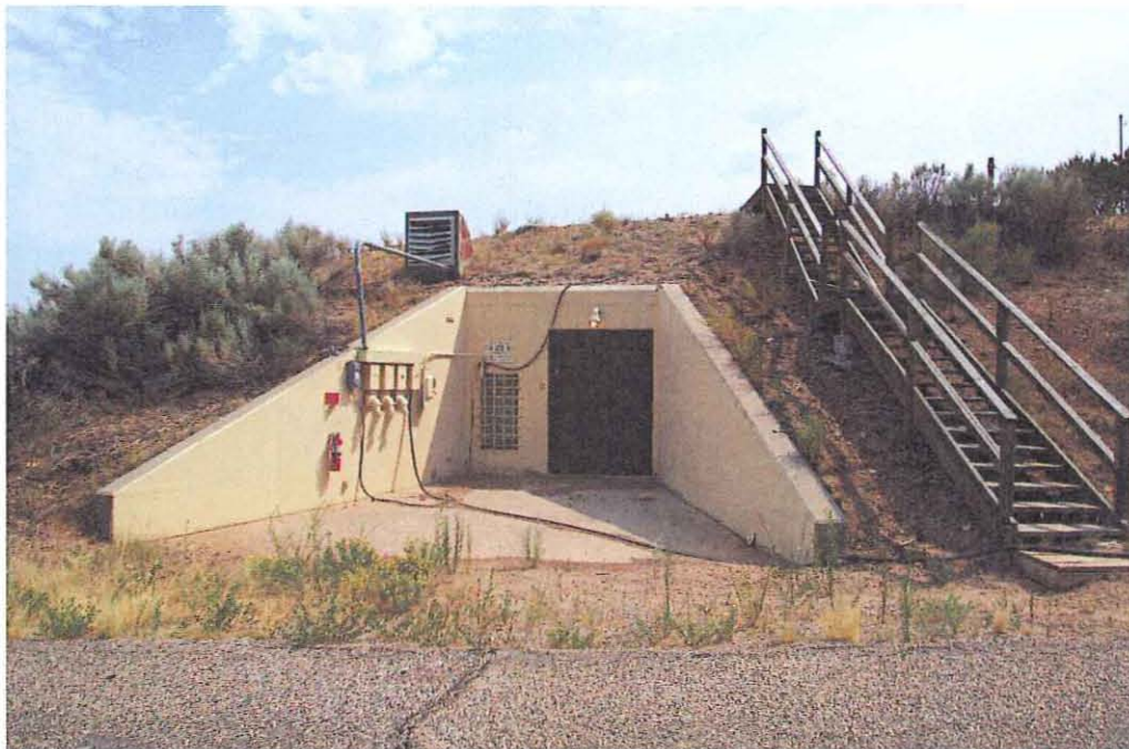
Fig. 8. Transformer Vault, TA-33-95
