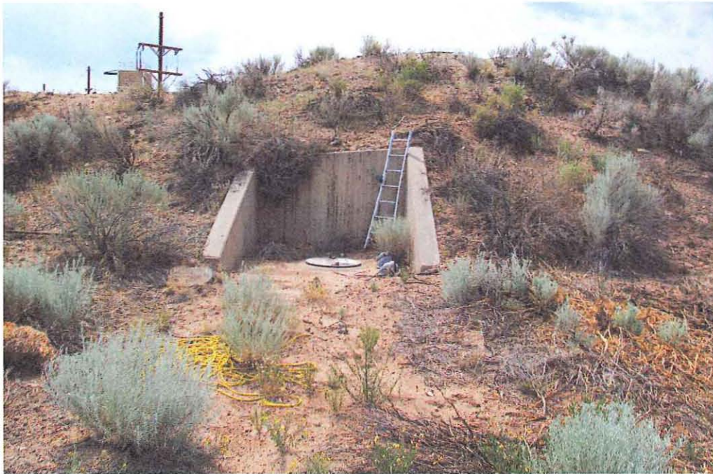
Fig. 7. Cable Tunnel Entrance with Manhole, Near TA-33-87
