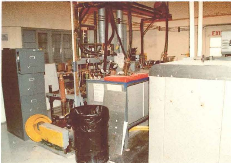
Figure 38. TA-21-12, Bay 5205, arc melter.
