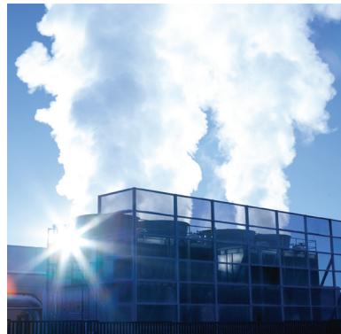
Cooling towers at the Los Alamos Metropolis Center for Modeling and Simulation dissipate the heat generated by the Laboratory's supercomputers.
