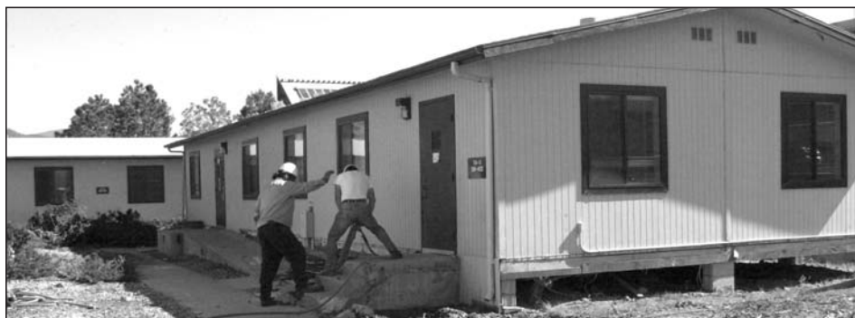
Work to prepare the buildings that formerly housed the Institute for Geophysics and Planetary Physics (IGPP) for removal stepped up earlier this month with construction workers jackhammering off entrance stairs. In addition, shrubbery was removed to accommodate getting the structures off site. Photo by LeRoy N. Sanchez
