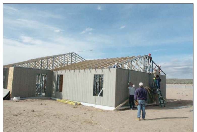
Top photo, Jerry Romero of Physical Chemistry and Applied Spectroscopy (C-PCS) fastens metal joists on a Habitat for Humanity steel frame home he helped build in Los Lunas in 2004. In the middle photos, Romero is on the roof of the home fastening an interior wall to an exterior wall. Bottom photo is a wide view of the same house under construction. Photos by Norm Daviess, Habitat for Humanity
