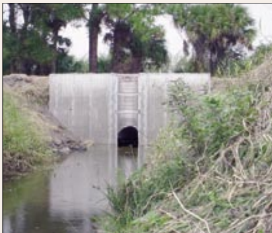
This riser board structure is an example of an improved water control structure that has been installed in citrus groves in Indian River County.
