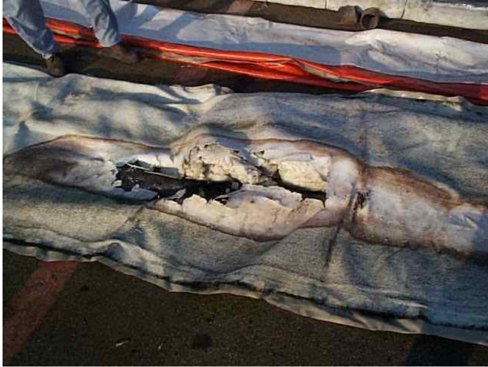
Figure 62 - Close-up of damage to felt layer with stainless steel mesh removed.
