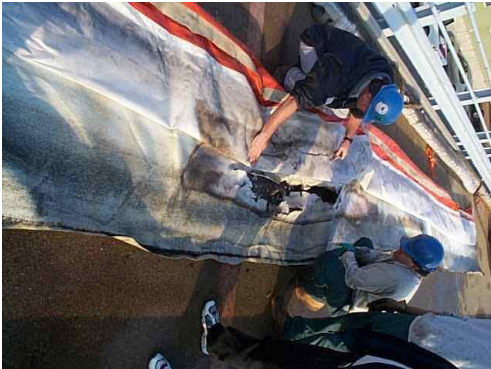
Figure 61 - Boom on deck showing damage to felt layer with stainless steel mesh peeled back.
