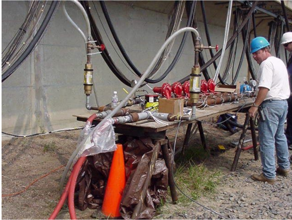
Figure 5 - Propane regulator bank and compressed air manifold valves.
