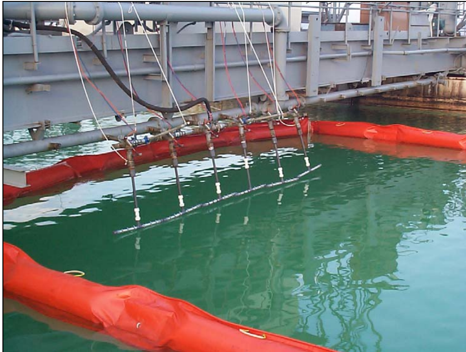
Figure 2-2: Oil Distribution System, October 2003.
