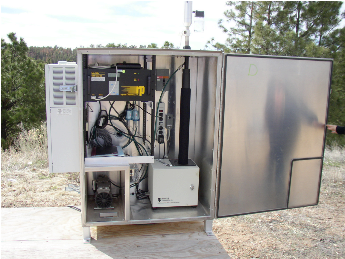
Figure 4-1. TEOM sampling equipment inside an enclosure at Site #61.
