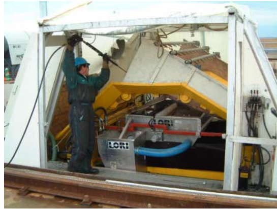
The LORI unit installed in the LGB. The three spraybars with nozzles are seen above the belt.
