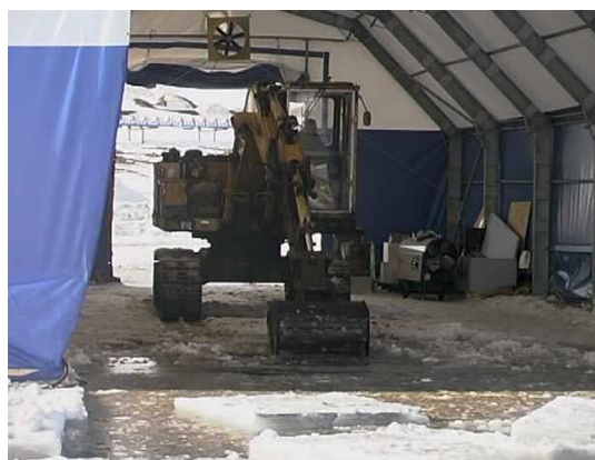
After assembling and launching the work platform, ice was removed inside the tent to allow the platform to float in.
