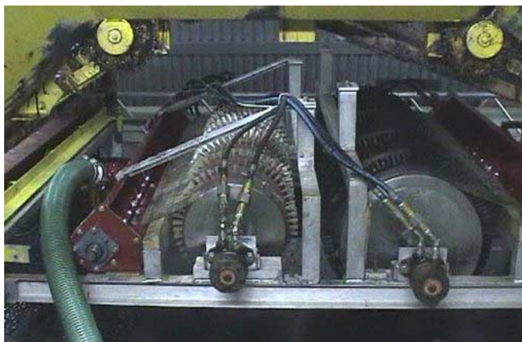
Figure 4.16 MORICE Brush-drum installed in the LGB.
