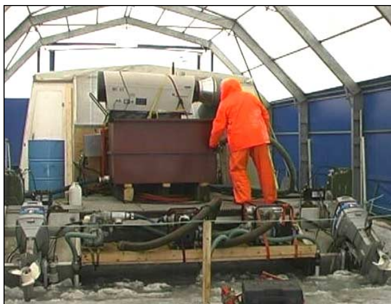
Figure 3.1 Water pumps on separate platform.
