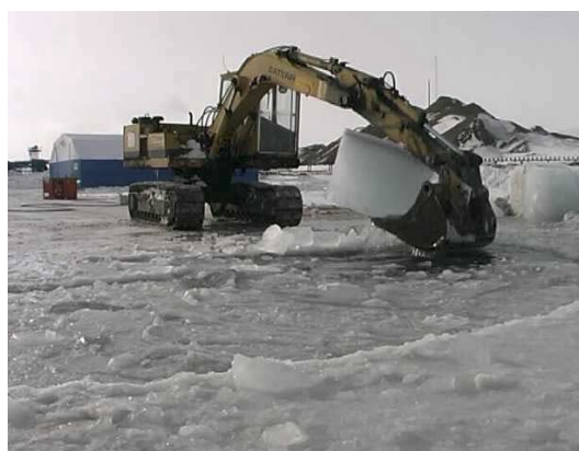
Removing ice from the circular end of the pool. The other end of the pool will be close to the tent.
