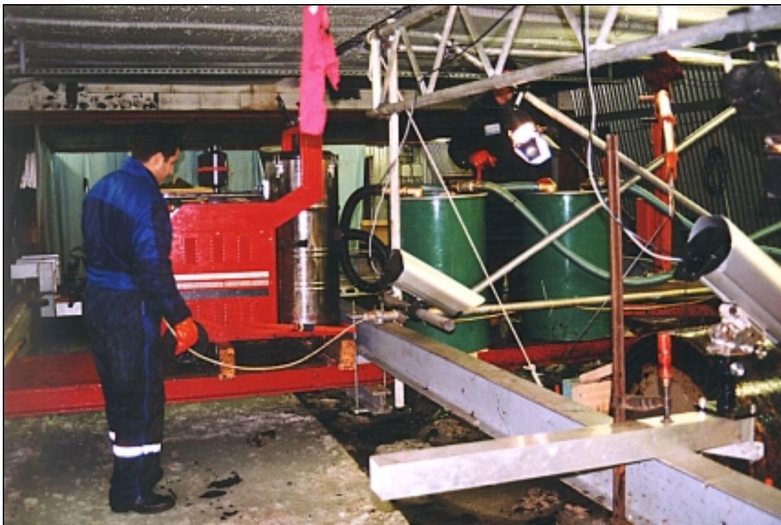
Secondary carriage with air conveyor and two barrels for recovered product, one for each of the two large drums.
