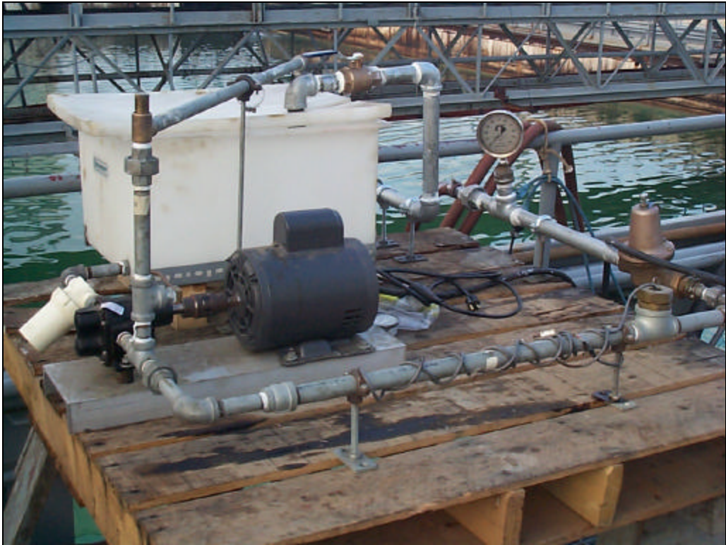
Figure 6. Dispersant Supply Tank and Pump
