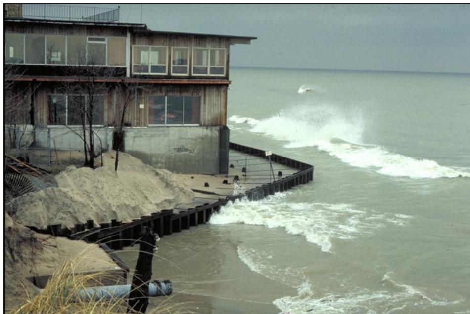
Figure 27. Shoreline erosion - Red Lantern Restaurant, Lake Michigan, Indiana. Photo courtesy of R. Royce, National Park Service, Indiana Dunes National Lakeshore, obtained from EPA Great Lakes web site.
