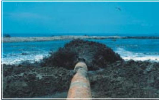
Dredged sand is pumped onto East Timbalier Island to stabilize, support and restore dune and marsh habitats after hurricanes created a breach in the island and compromised island habitats.
