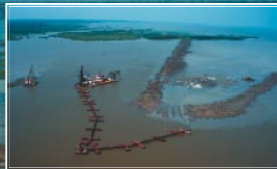
Mid-stage construction creates a suitable platform for new delta habitat, Big Island, Louisiana.
