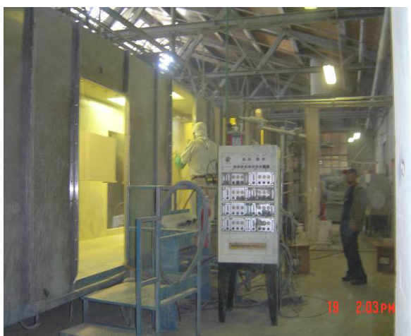
Figure 1. Powder paint spray booth
