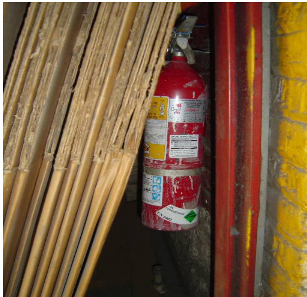
Figure 6. Fire extinguisher blocked and hidden by boxes.
