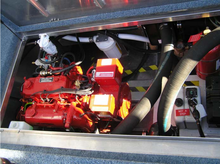
Figure 1. Westerbeke Low CO Generator (top) and Catalytic Air Pollution Control Device (bottom).
