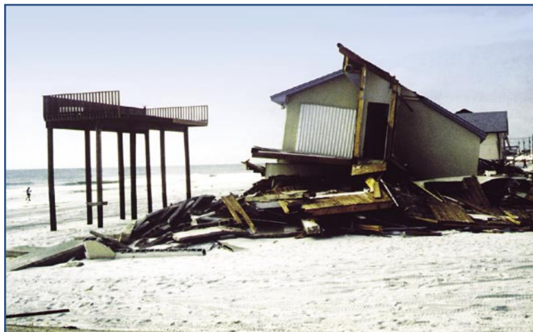
Damage from Hurricane Opal in Florida. This deck was designed to meet State of Florida Coastal Construction Control Line (CCCL) requirements. The house predated the CCCL and was not.
