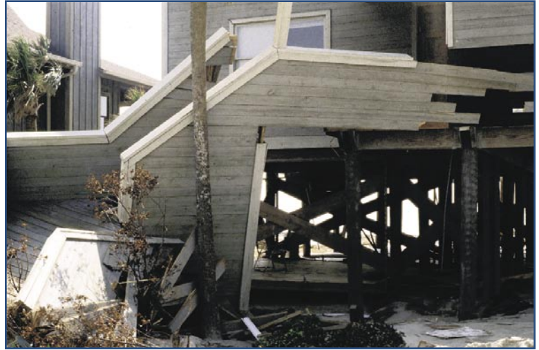
The rails on these stairs were enclosed with siding, presenting a greater obstacle to the flow of flood water and contributing to the flood damage shown here.
