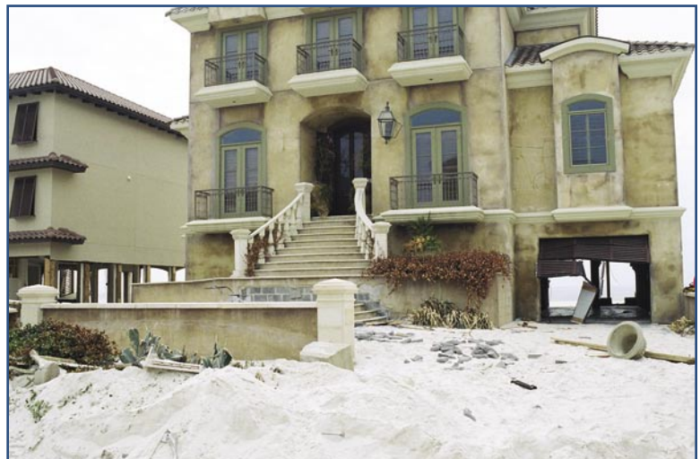
Large solid stairs such as these block flow under a building and are a violation of NFIP free-of-obstruction requirements.
