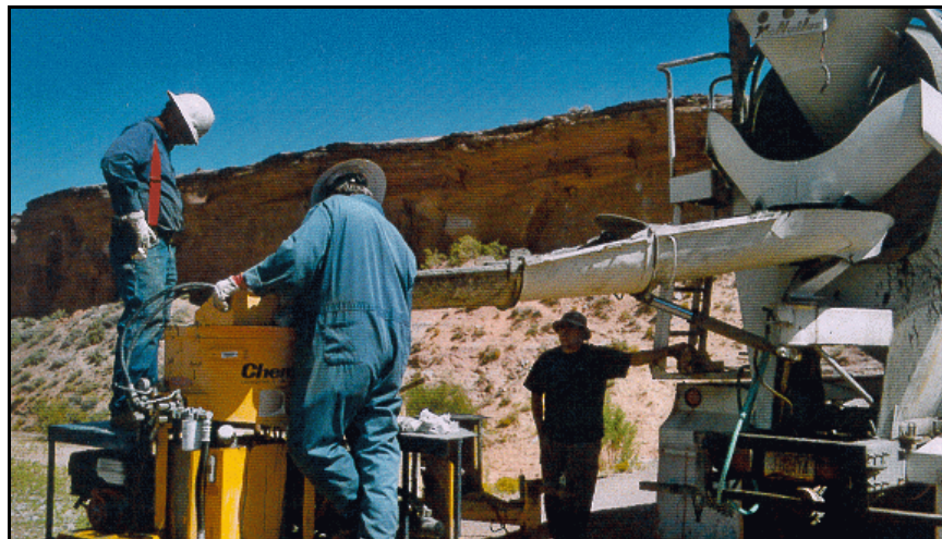
Figure B-62. —Grout mix being conveyed directly into the grout mixer from the transit mixer truck.
