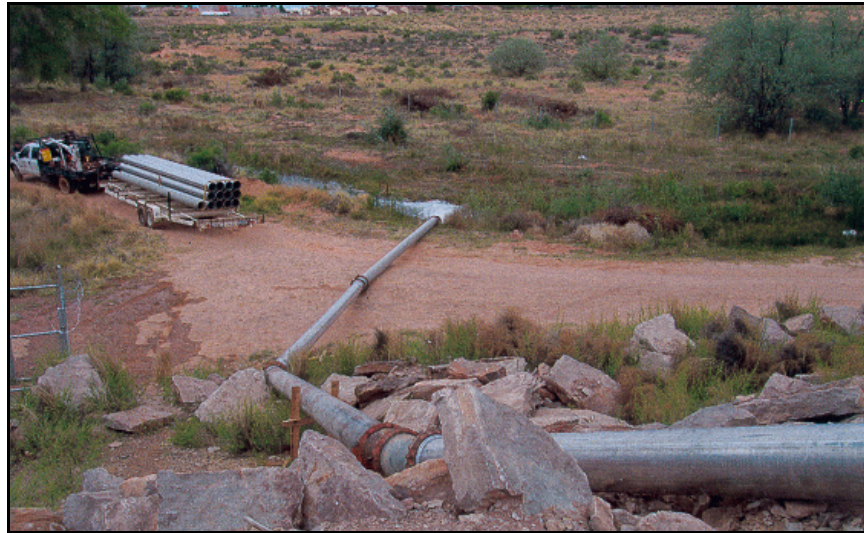
Figure B-61. —Siphon constructed over to crest of the embankment dam for discharging irrigation releases.
