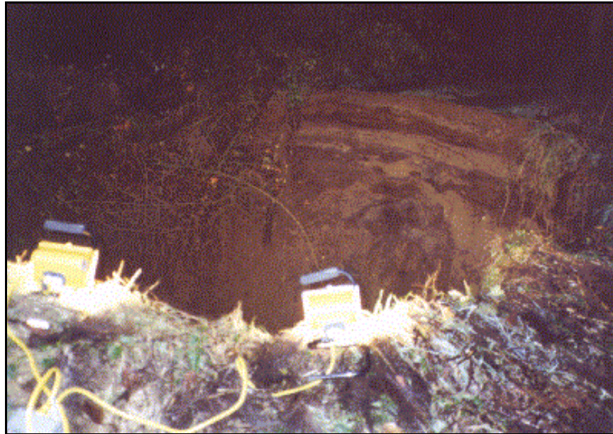
Figure B-56. —Sinkhole in the dam crest the night of December 11, 1996.
