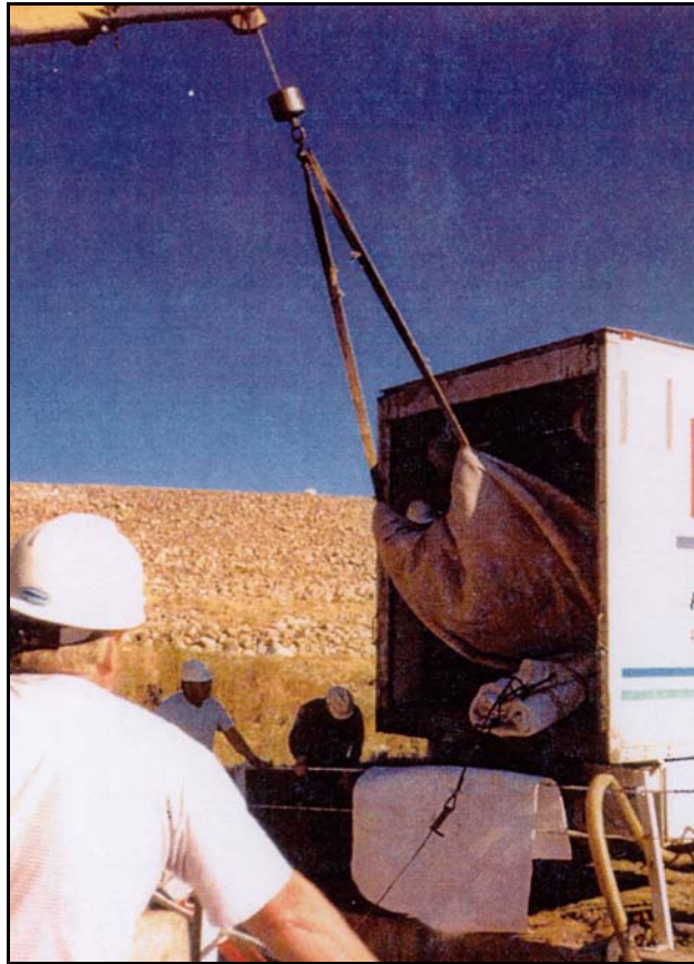
Figure B-80. —Lowering of the CIPP liner into the stilling basin, so it can be winched up the tunnel.
