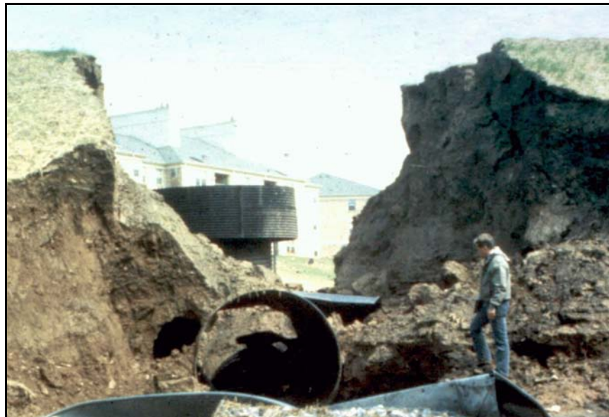
Figure B-51. —Loveton Farms Dam after failure as viewed from the downstream end of the 78-in diameter CMP spillway. Note that one of the antiseep collars, which were about 14 feet square, is visible in the breach.
