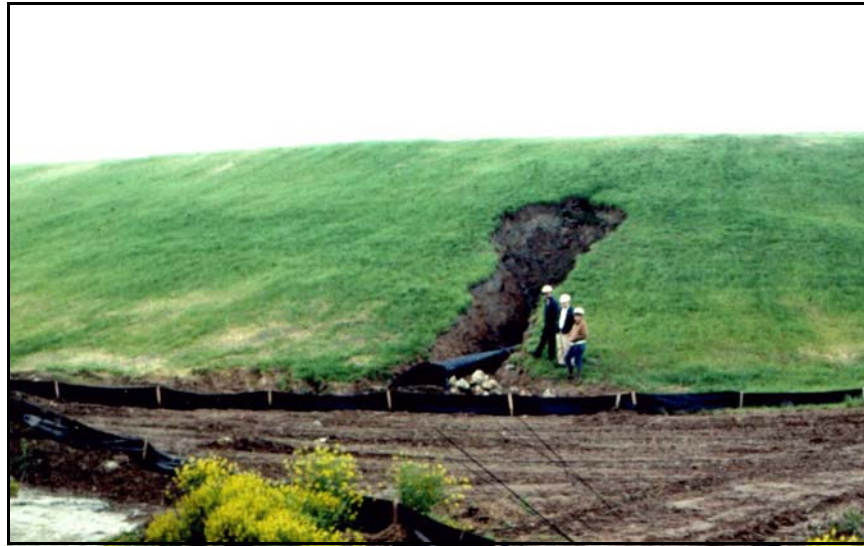
Figure B-55. —When the pool level of this embankment dam was only about 2 to 3 feet deep, flow along the outside of the CMP resulted in loss of the adjacent soils.
