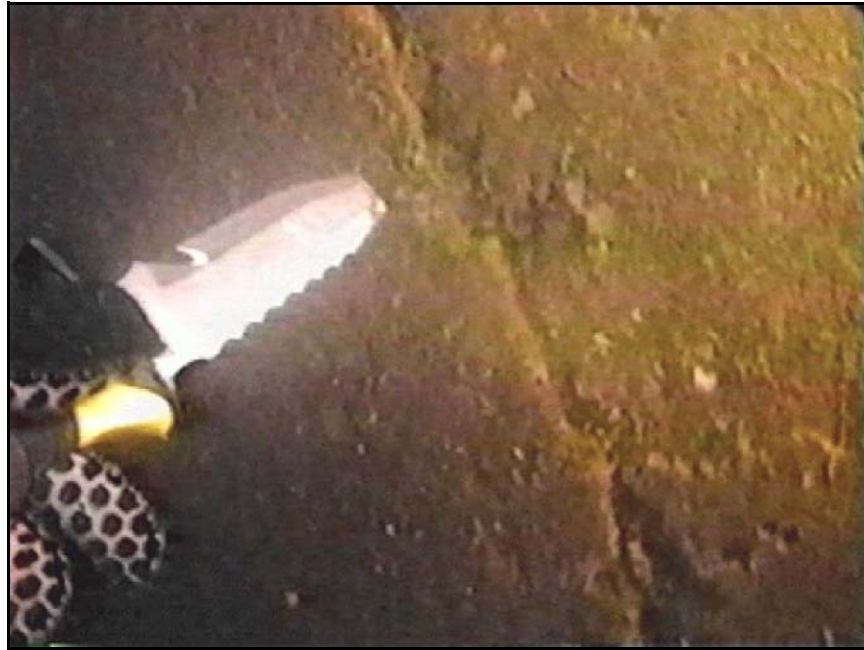
Figure B-73. —The diver used a knife to probe cracks in the concrete. Divers prefer knives with blunt ends in underwater inspection, since it is less likely that a hole could accidentally be poked into their dry suits.
