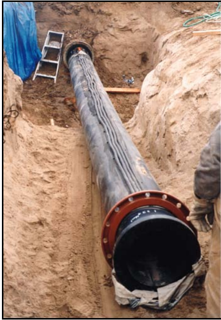
Figure B-75. —HDPE slipliner being installed at Turtle (Twin) Lake Dam. Note the HDPE grout lines welded onto top of new liner. The end flange was used to attach the two different sized liners together.
