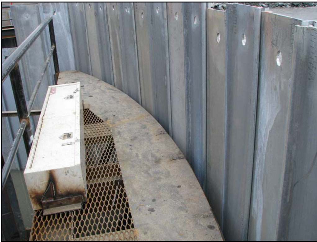
Photo 24. Template with a full set of sheet pile. Template curvature matches design curvature of cell face.
