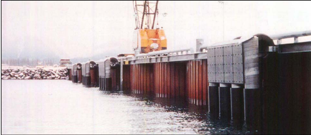
Photo 11. Example of open cell sheet pile dock and fendering systems.
