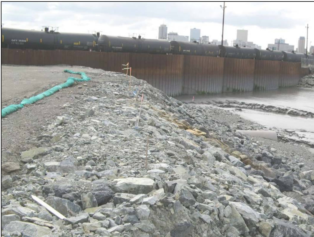
Photo 12. Flint Hills sheet pile wall looking along South Backlands dike to “tie in” point.
