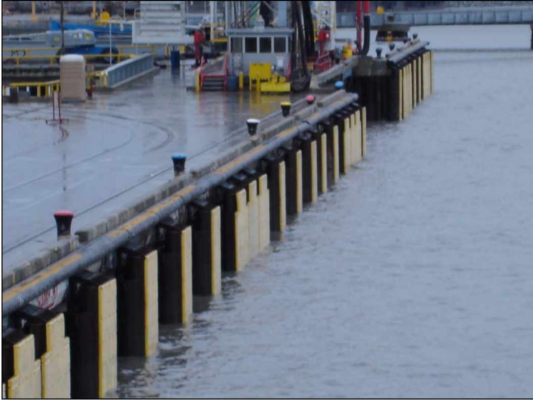
Photo 29. Existing fender system at the Port of Anchorage. New fenders will be similar.
