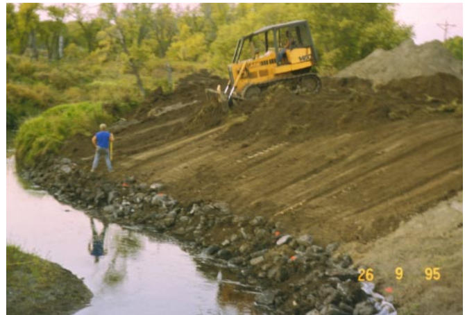
September 1995: A dozer moves dirt to begin reshaping the riverbank that had been eroded into a sheer cliff about 12 feet high. In 10 years, the riverbank had eroded 40 feet. Photo courtesy of Rich Axvig, NRCS.
