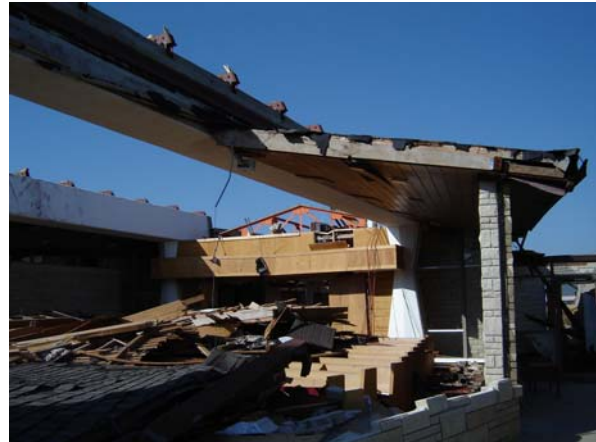
Figure 4: Laminated Roof Beam Failure
