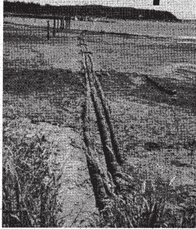
Saltwater pipelines serving the research laboratory.
