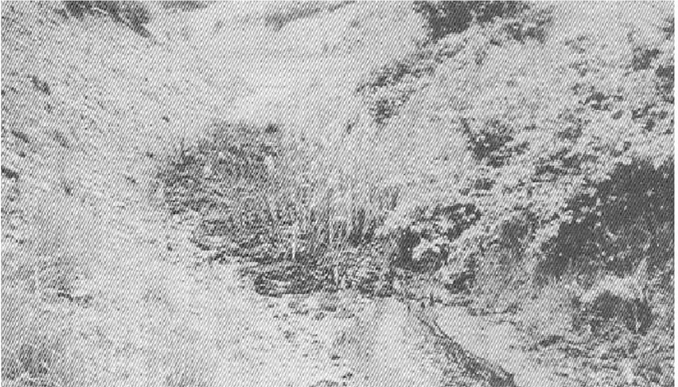
A Slide of Refuse Material and Vegetation Partially Blocking Diversion Ditch
