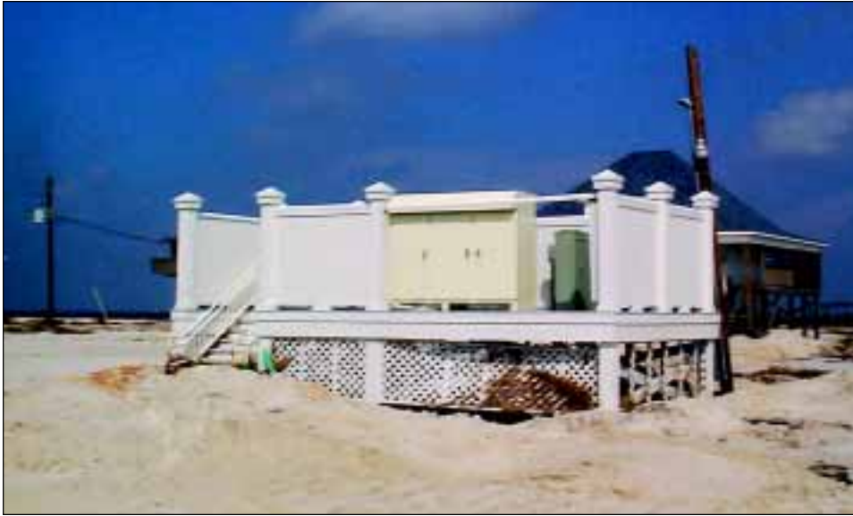
FIGURE 4-20 Other than losing part of the lattice screening, this elevated utility platform performed well.
