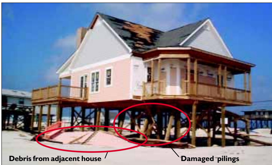
FIGURE 4-17 Damage to piles of a newly constructed house caused by impact of waterborne debris from a nearby collapsed deck.
