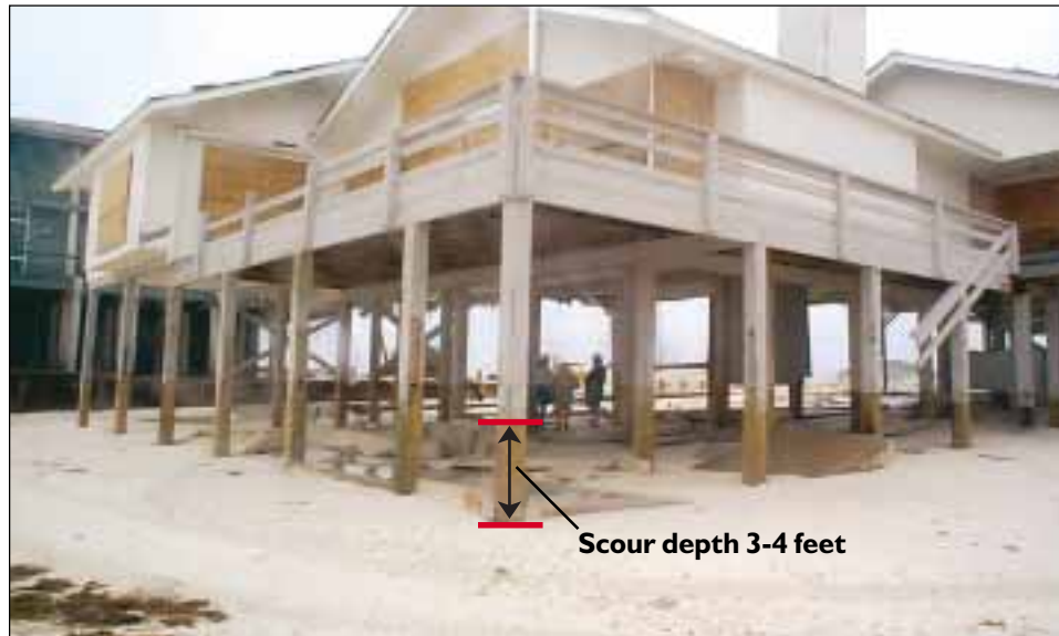
FIGURE 4-25 Despite the loss of 3 to 4 feet of sand, this structure performed well. Note at-grade slabs broke away as intended.
