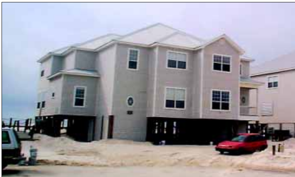
FIGURE 4-39 Fiber-reinforced concrete siding suffered no damage.
