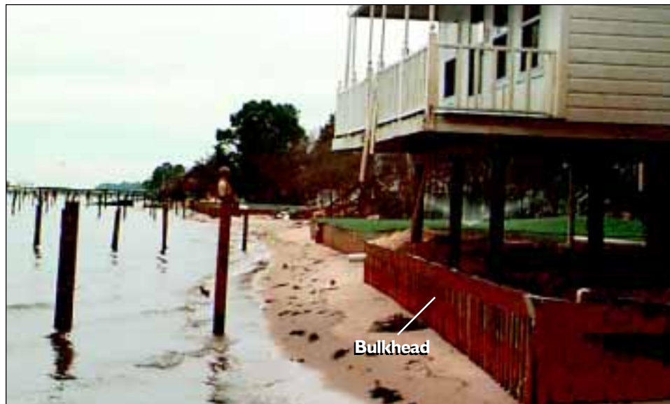
FIGURE 4-30 Bulkheads on Mobile Bay still in place after storm.
