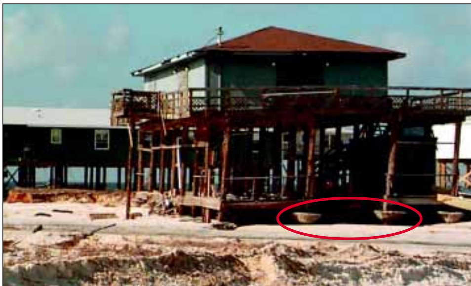
FIGURE 4-14 This house suffered pile settlement due to scour around piles with concrete collars. In addition, note the loss of stairs and damage to lower-level enclosed area.
