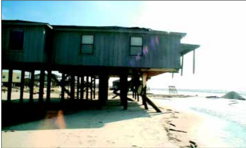
FIGURE 4-11 This house lost its deck and sustained structural damage to the Gulf side of the house.
