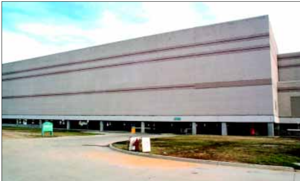
FIGURE 4-8 The area below the BFE is used for parking and required only minor clean-up following the flood.
