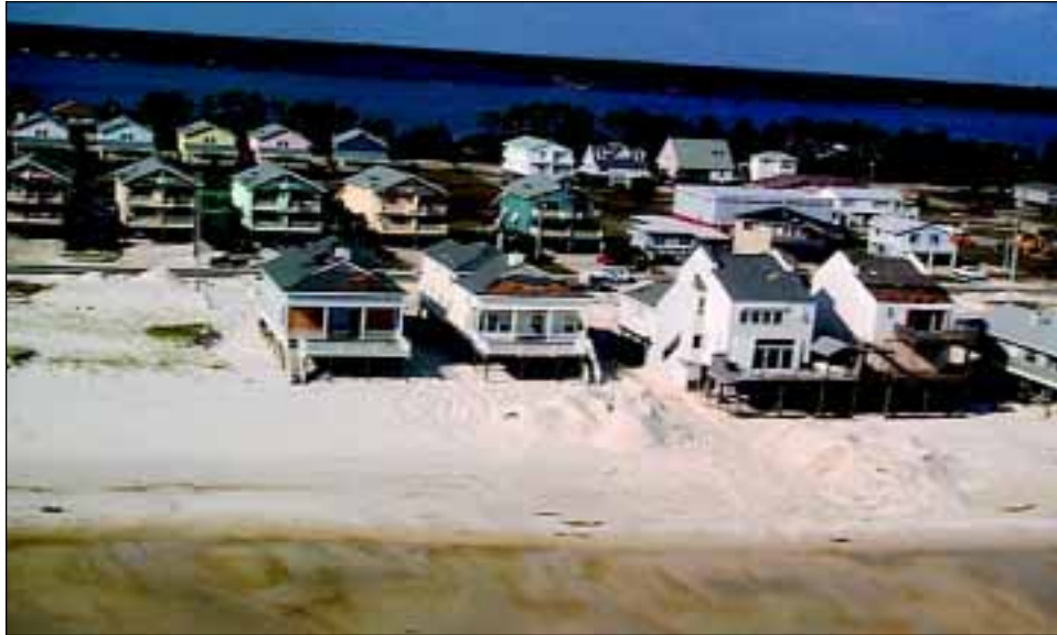
FIGURE 4-36 Houses in Gulf Shores with roof damage. Note loss of roof covering on front-row buildings.
