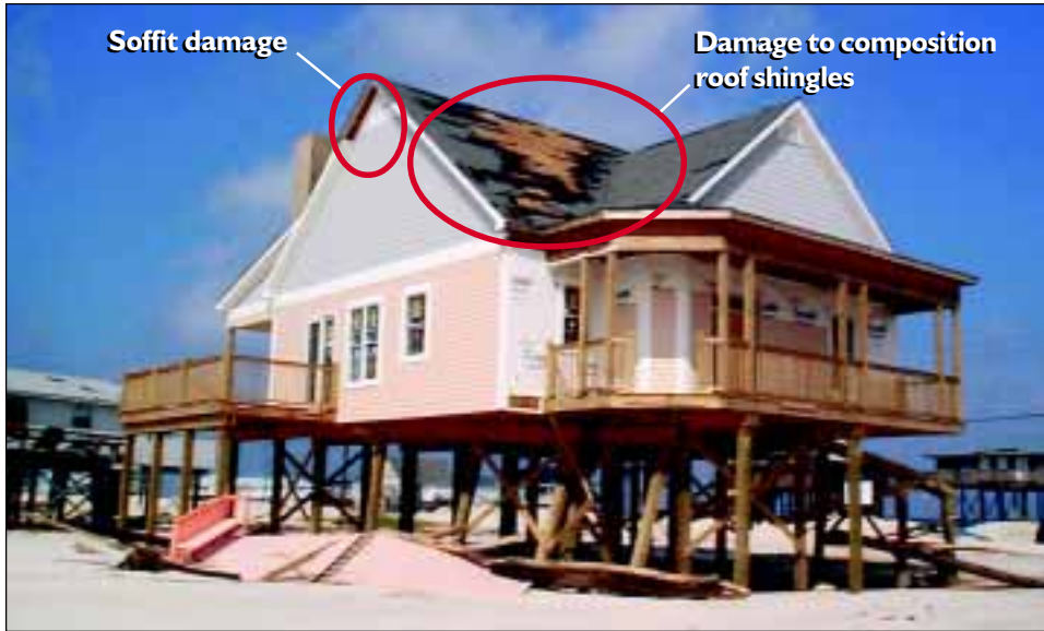
FIGURE 4-34 Wind damage to composition roof shingles and siding on newly built coastal home.
