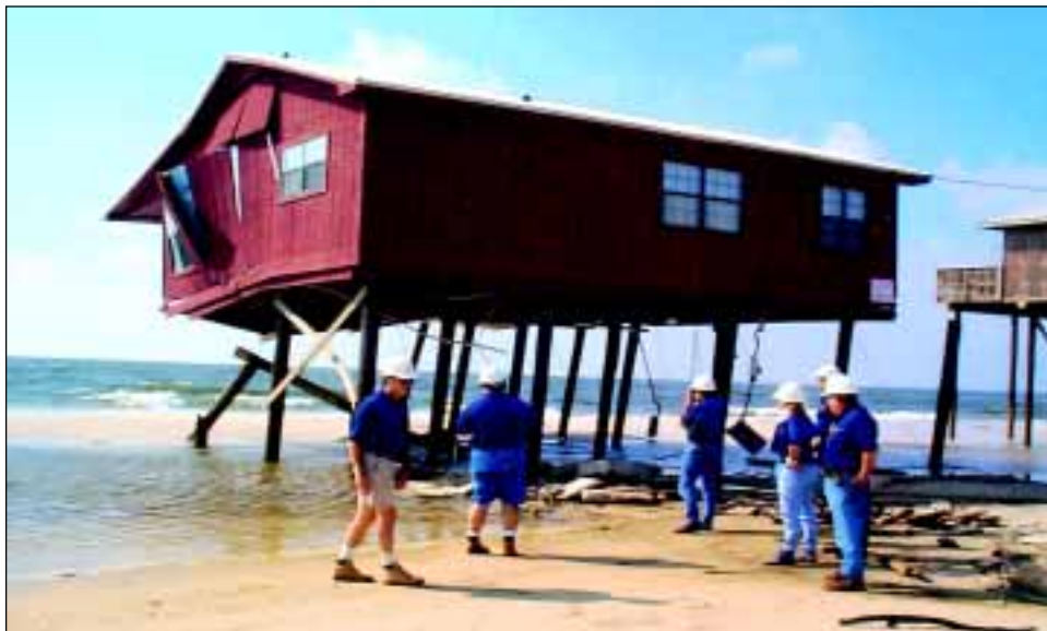
FIGURE 4-12 The BPAT observing a partially collapsed front-row structure.
