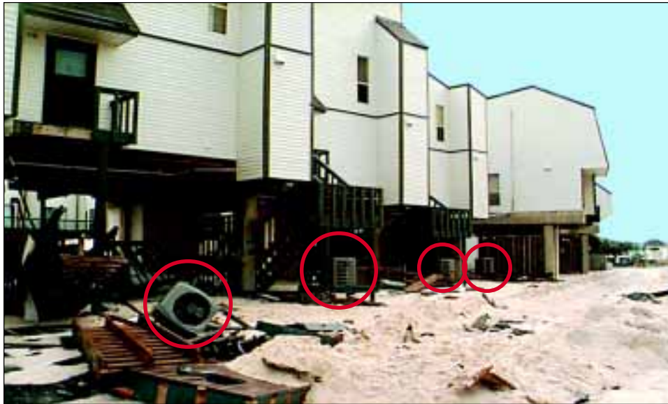
FIGURE 4-23 These air conditioner/heat pump compressors in Gulf Shores were not elevated and therefore were severely damaged.
