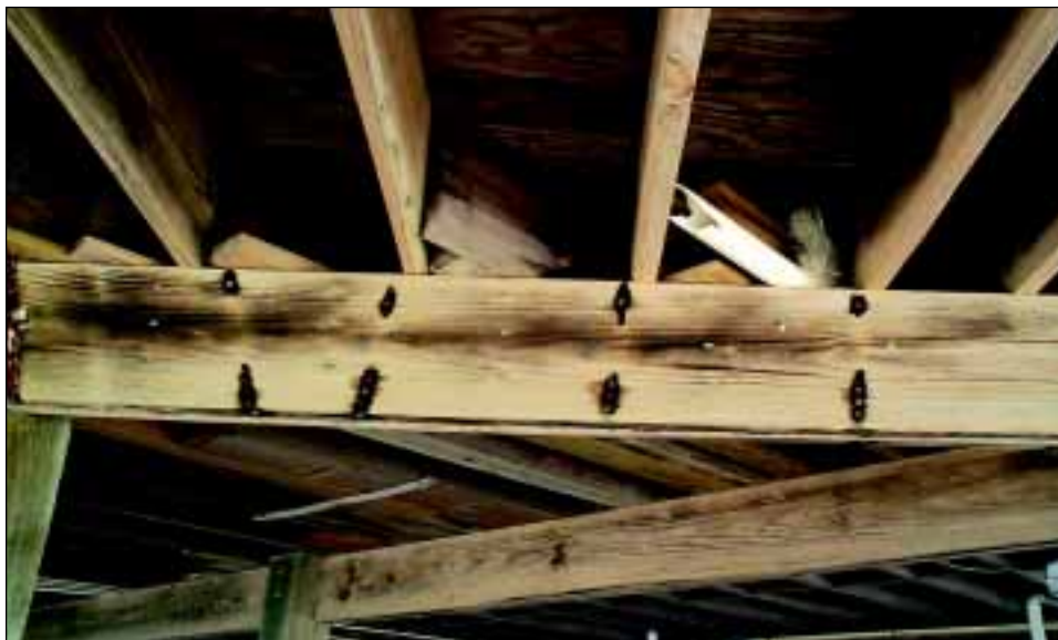
FIGURE 4-24 Only remnants of corroded hurricane straps remain.
