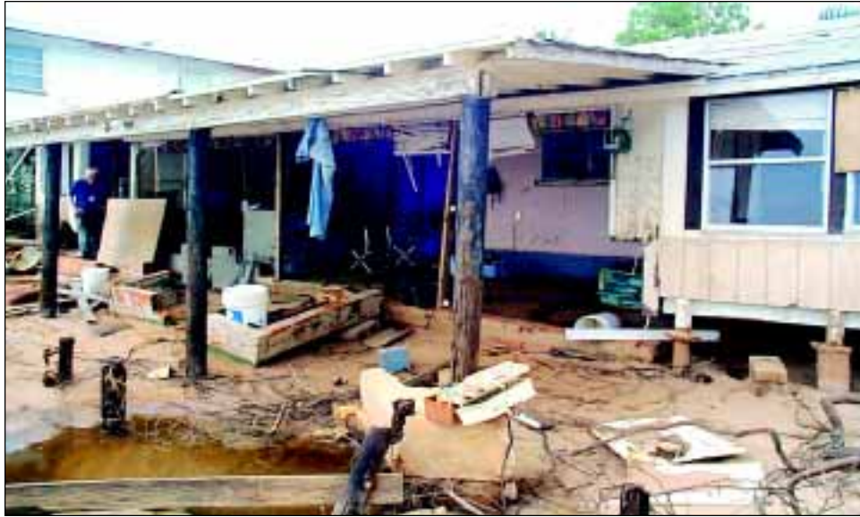
FIGURE 3-8 In some cases, scour behind bulkheads resulted in structural damage along Mobile Bay, Alabama.
