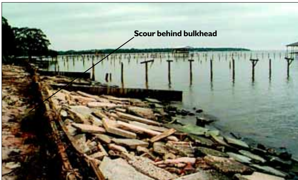
FIGURE 3-7 Remnants of fishing piers in Mobile Bay near Fairhope, Alabama. Note scour behind the bulkhead on the left.
