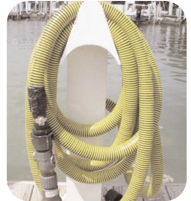
Using a pump-out station to properly dispose of sewage is one way boaters can reduce nutrient inputs to nearshore waters.
