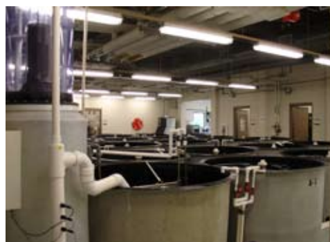
Advanced filtration systems allow reuse of seawater.
