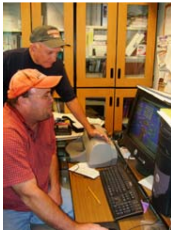
Cleve and Kevin on the Johnson control panel. The on-site engineering team sustains environmentally-friendly operations is less costly than paying excessive energy and water bills.
