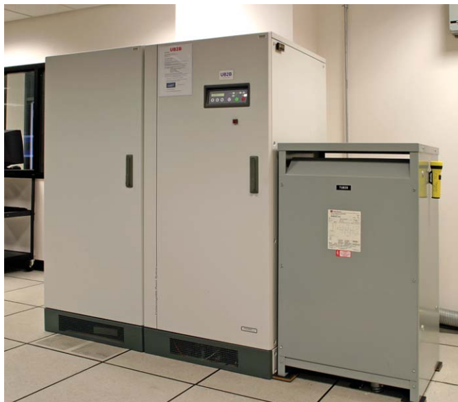
Figure 11. The new 100 kVA Chloride Uninterruptible Power Supply in FSL Central Facility.
