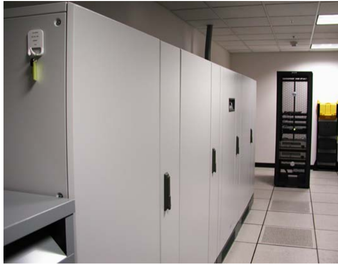
Figure 10. Uninterruptible Power Supply (cabinets to the left) and the GOES ground-station rack (tall, black unit toward the back) in the new Central Facility Annex.
