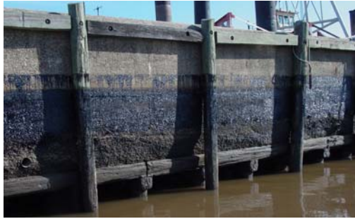
a. Oiled seawall
