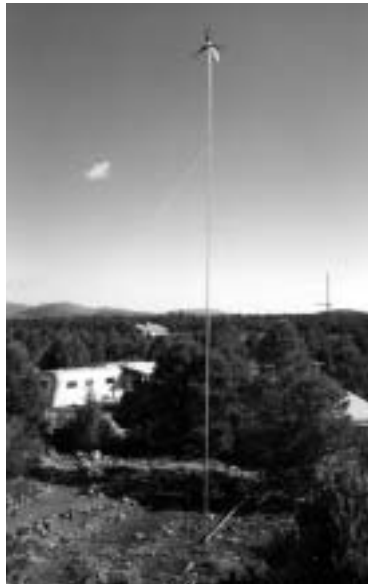
A Southwest Windpower Air 303, 300 watt turbine is the sole source of electricity for this remote home in northern Arizona.
